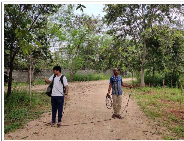
Figure 5.2: Providing power connection in Botanical garden
